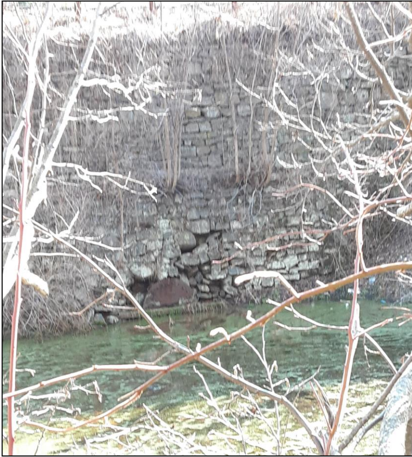
Loose stones around outlet pipe
