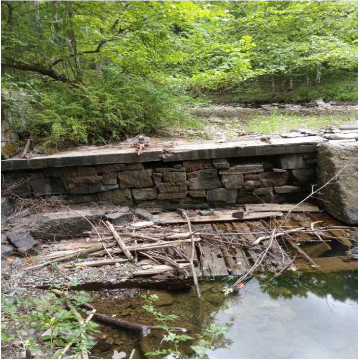
Old photo of Northwest abutment when it still had the capstones. Only one capstone remains today.
