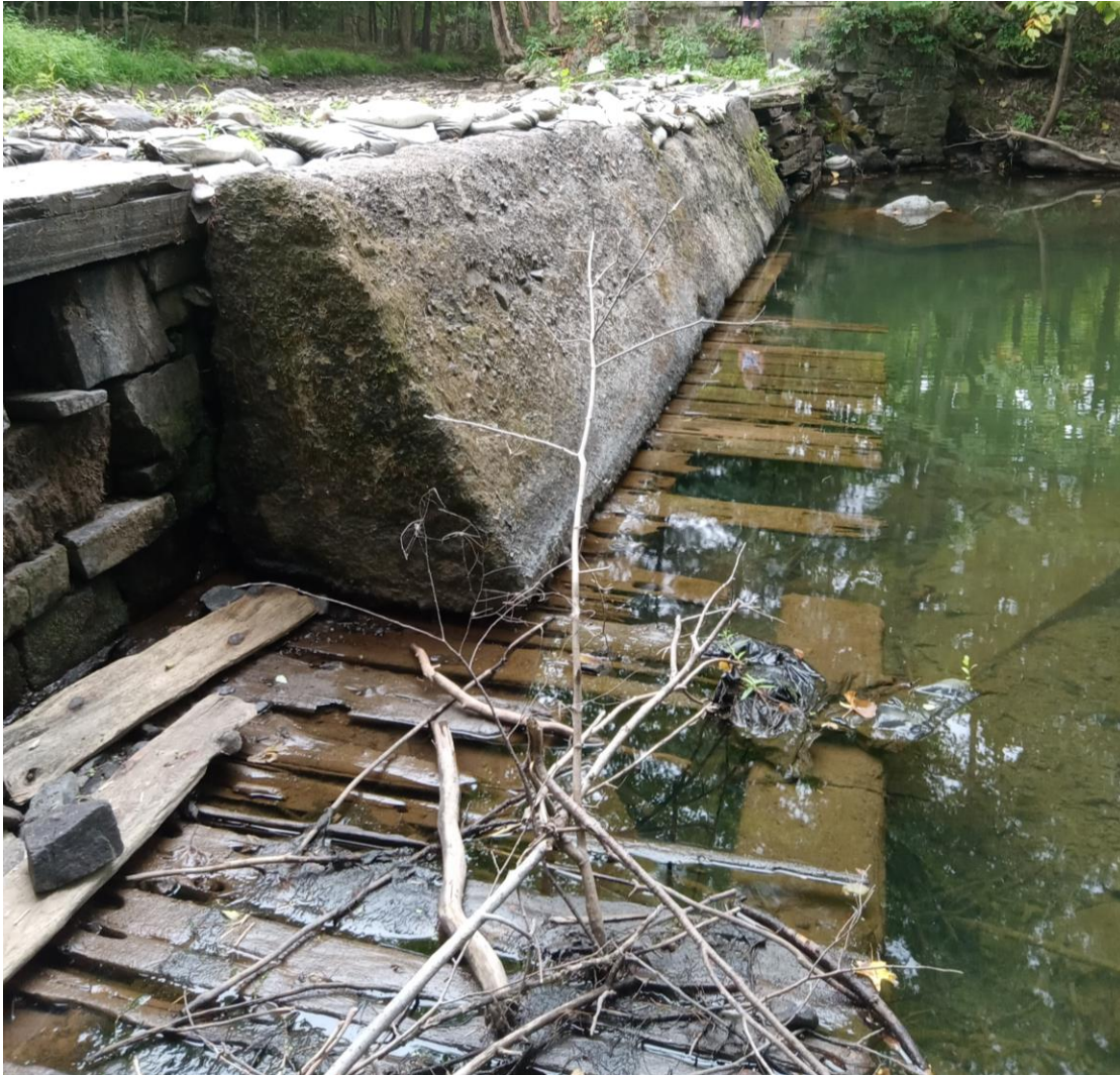
Weir photos were taken during drought of 2022 revealing the deteriorating condition of the structure including rotting boards underneath the Weir.
