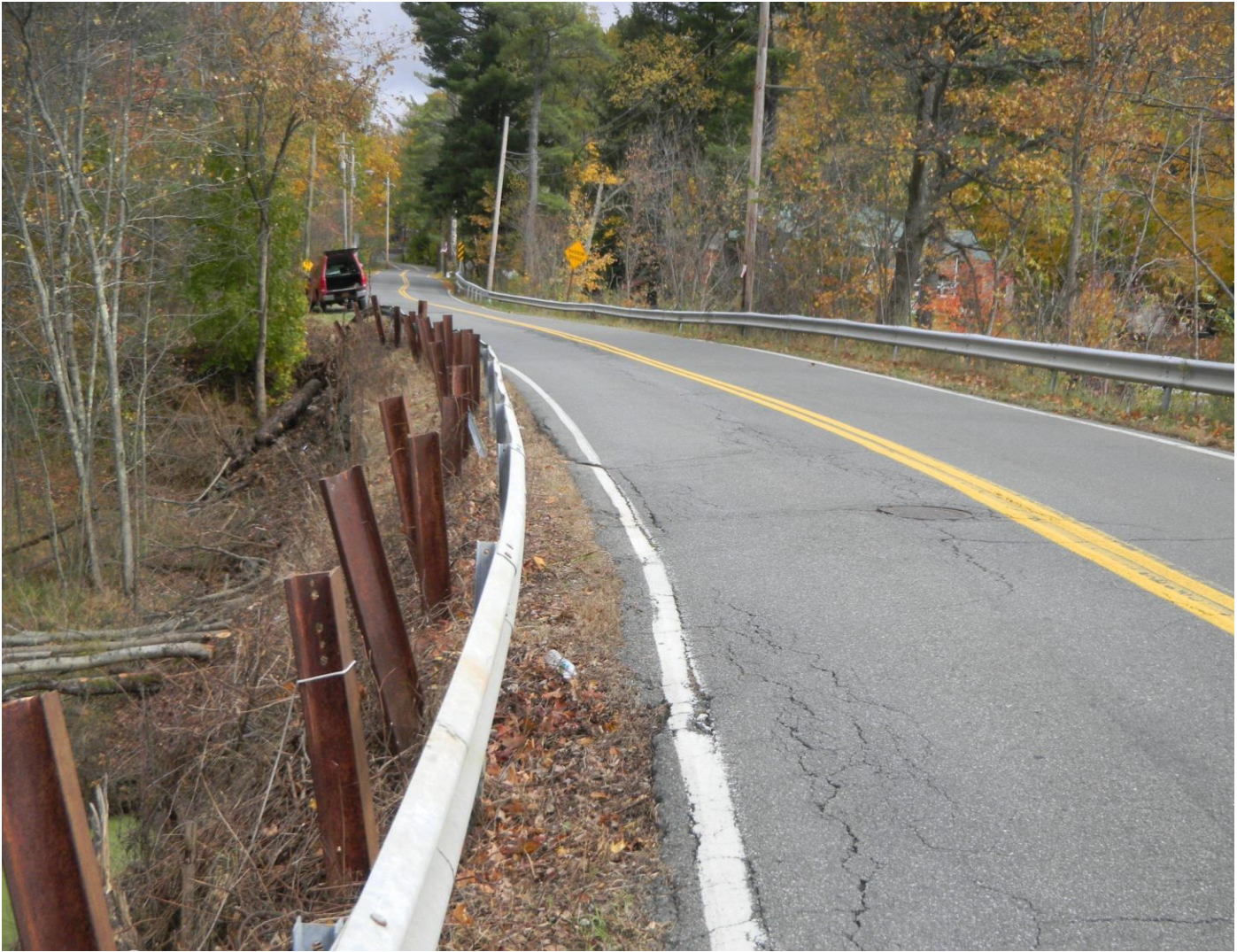
There are many Stress cracks in the road on top of the dam
