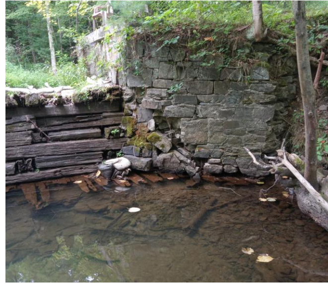
Above - Southeast Abutment Left – Northwest Abutment Both falling apart!
