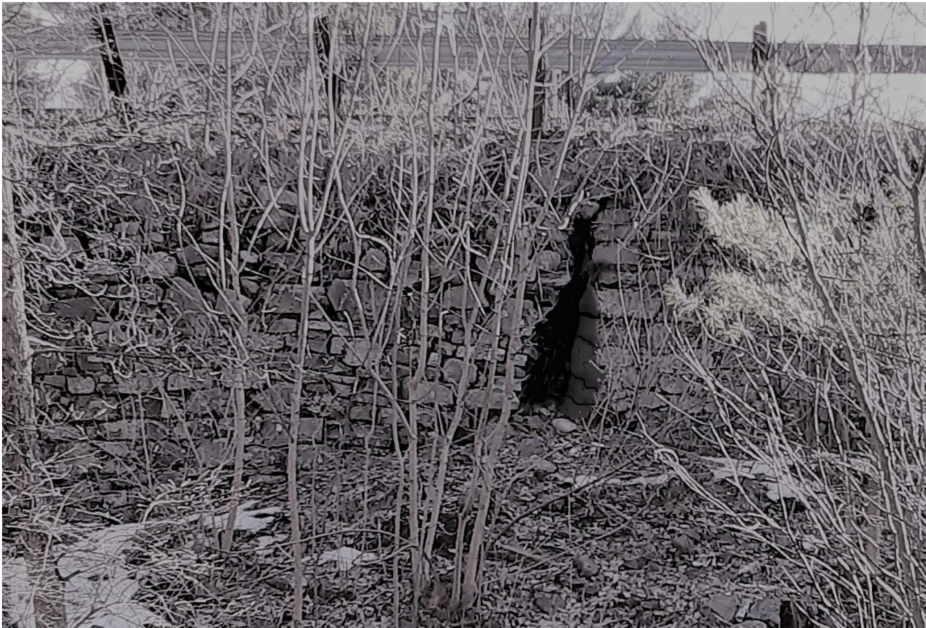
6' Hole in face of wall. Stones left of hole appear to be collapsing.
