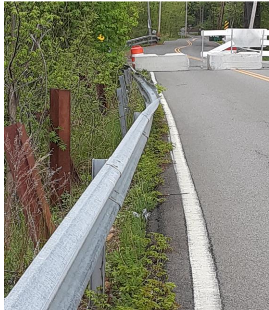
Road closed, guard rails and supports separated and unstable.
